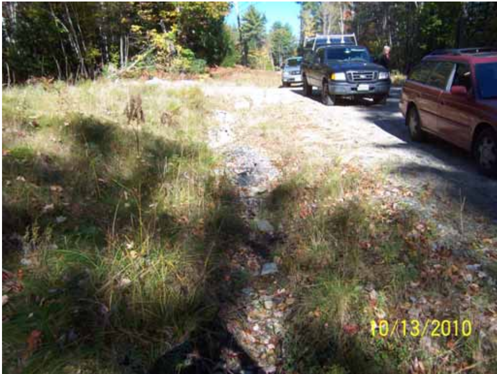
13. Erosion noted in ditchline adjacent to Wildwood Road
