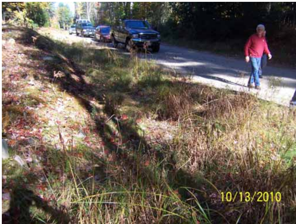
14. Eroded/exposed cut bank adjacent to ditchline along Wildwood Road
